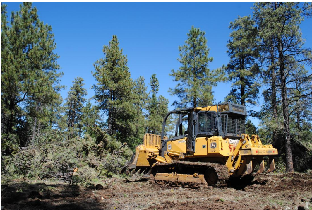
Dozer Operator, Lee Payne, continues prep work ahead of the burn in the McCracken East project area south of Williams, AZ along County Road 73.
