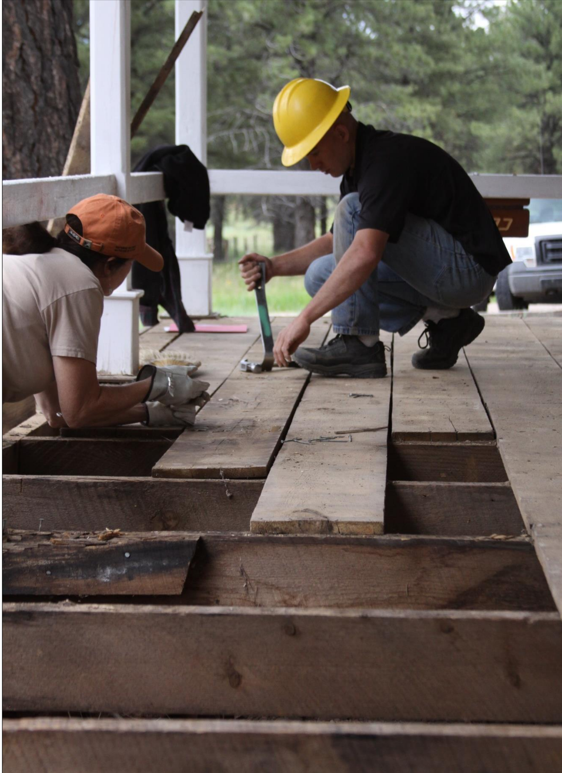
Porch demolition on Jacob Lake Ranger Station cabin restoration project, July 2015. Photo by David Hercher. Credit the U.S. Forest Service, Southwestern Region, Kaibab National Forest.
