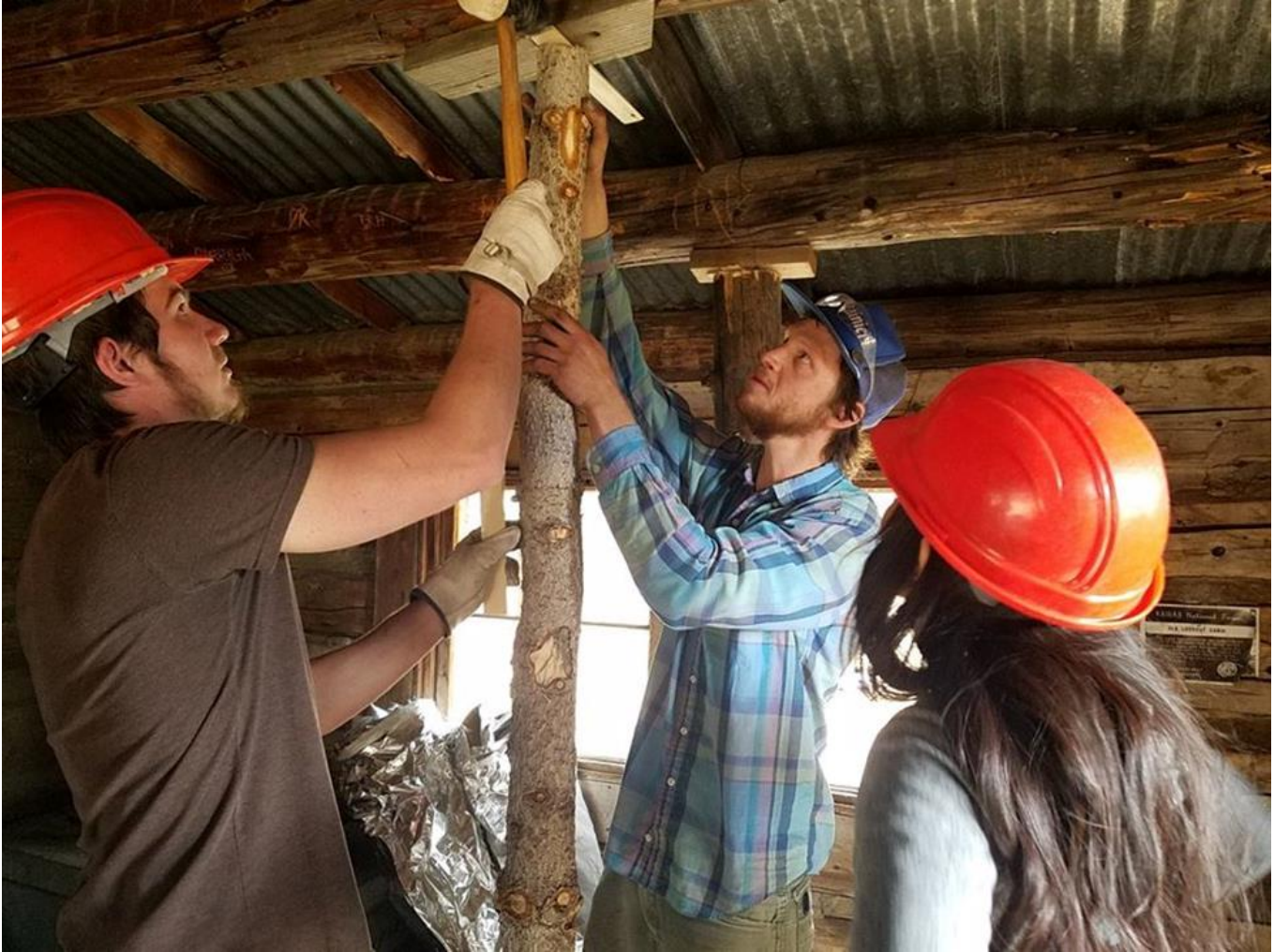
Students from Dr. Lee's fall 2017 Wilderness Management class adding support beams to stabilize the damaged roof at Kendrick Mountain Cabin. Credit Kaibab National Forest.
