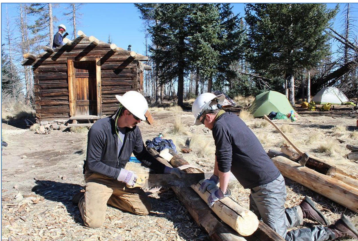
Kaibab National Forest employees, partners and volunteers have worked together for more than two years to rehabilitate the historic 1911 Kendrick Mountain Fire Lookout Cabin. Photo courtesy Neil Weintraub.
